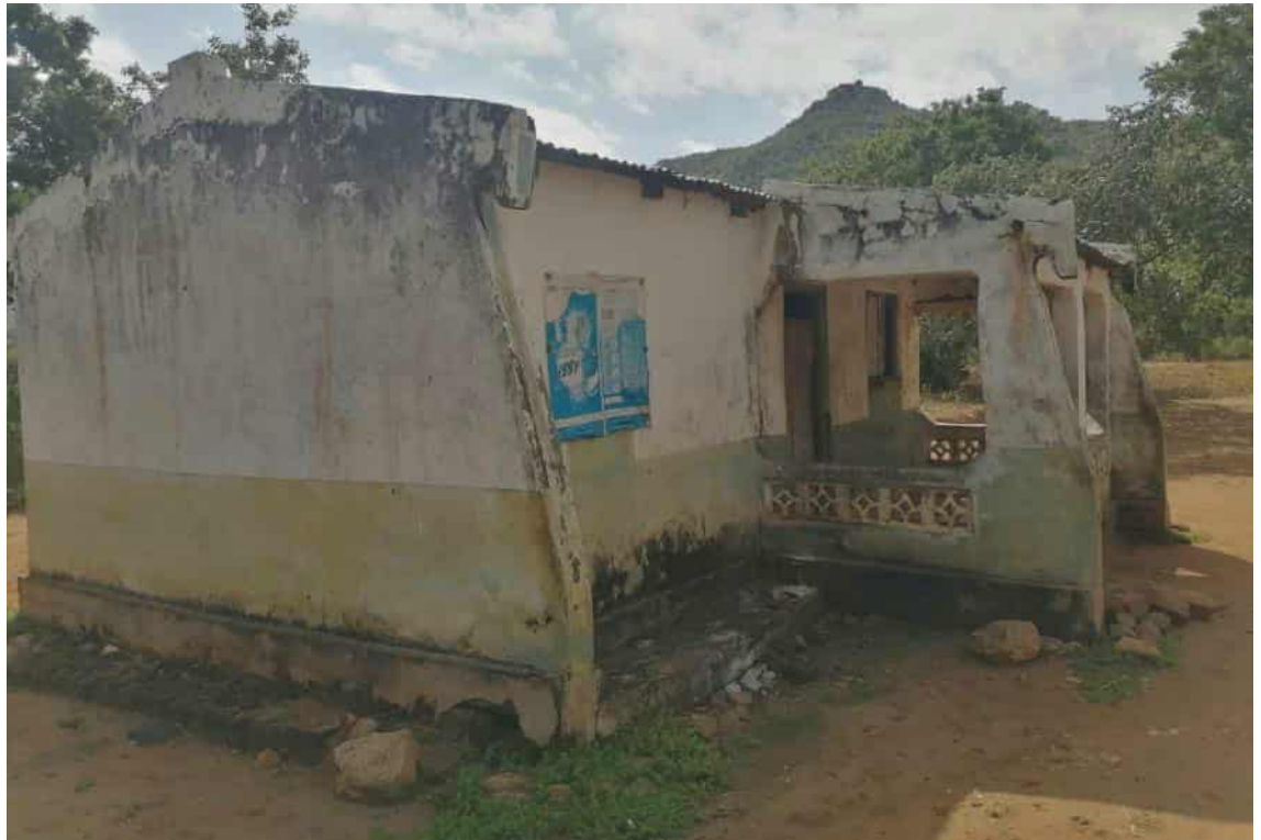
H8 Burnt bricks - cement floor - plastered inside and outside - corrugated iron sheets
